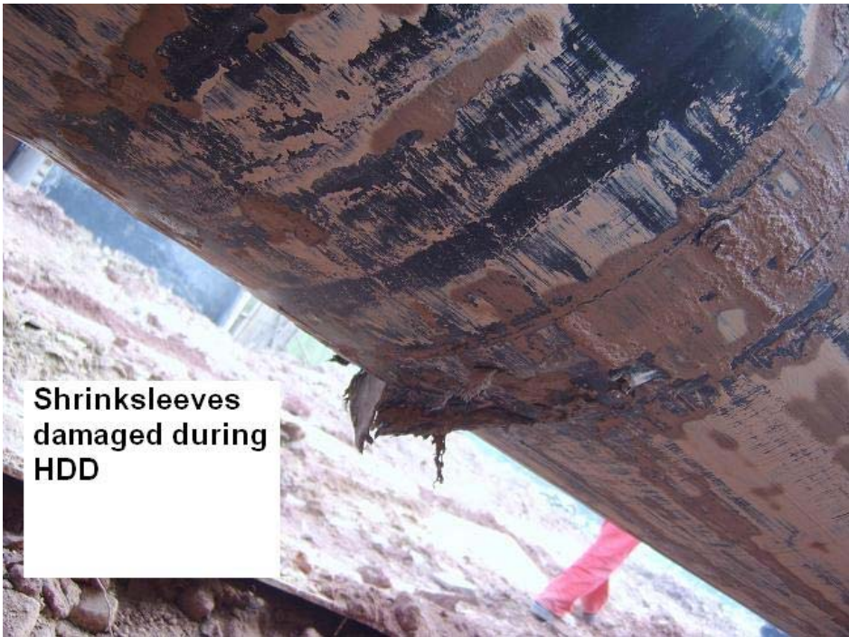
Figure 5A – Shrink sleeves used on the 3 LPE coated pipes in the HDD BP's Quandong LNG Dapeng Project China
